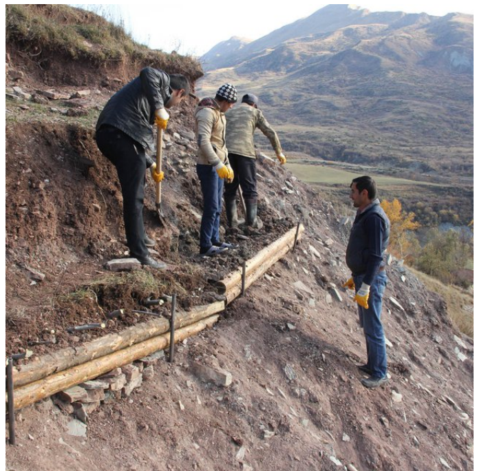
Construction of a pile wall on a steep slope in the village of Goydan (Hanns Kirchmeir)
